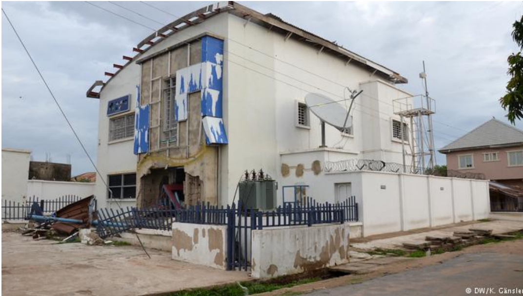
Boko Haram has left a lot of destruction - as in the small town of Mubi
